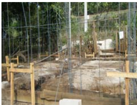
4. Place the rebar cages in the footings and the vertical rebar rods and corner cages.
