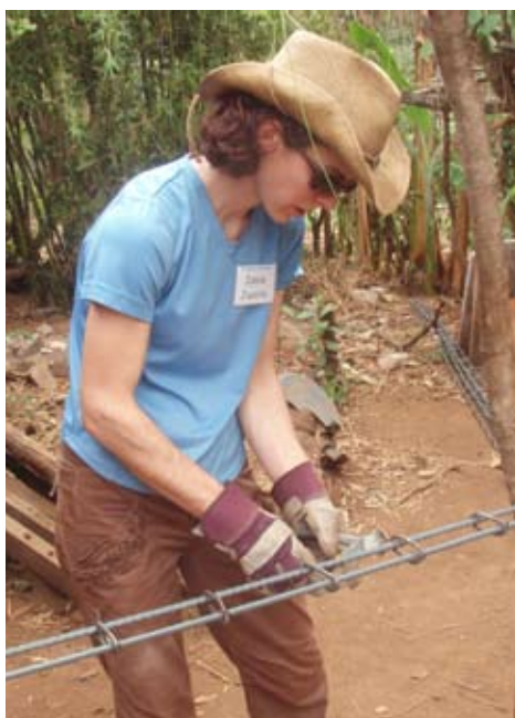
3. Prepare the rebar cages that will be used to re-enforce the house.
